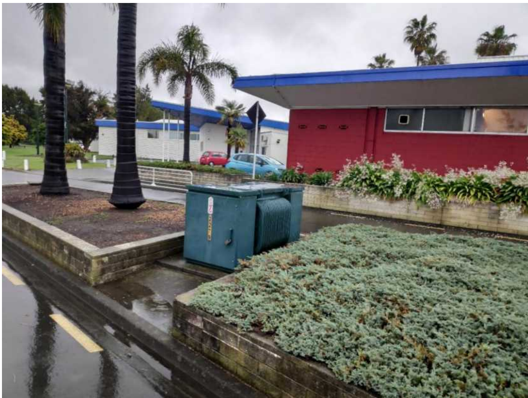
Photograph 8: An example of the electrical transformers observed onsite.
