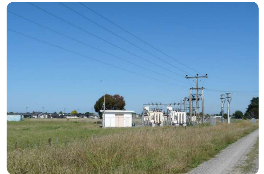
Existing Unison Networks Sub-Station
