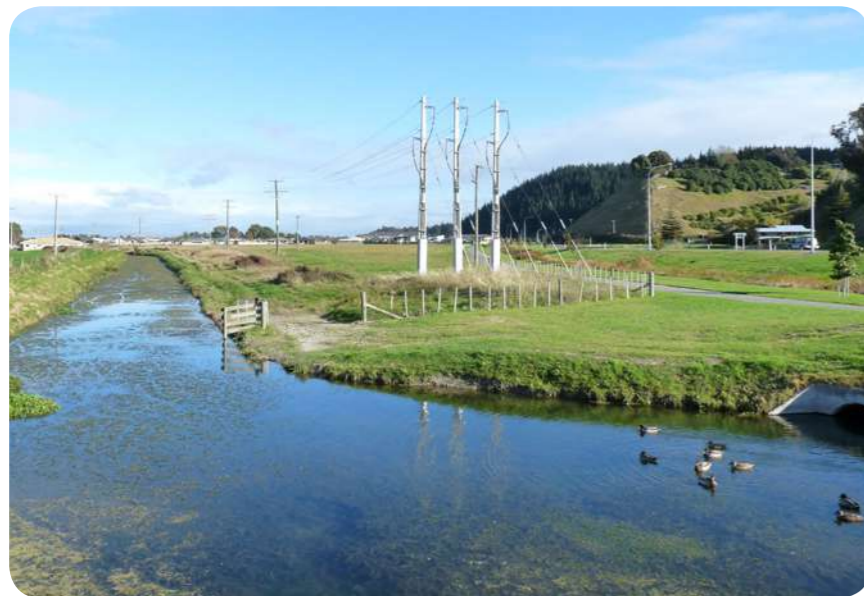
Overhead Lines near Taipo Stream (2013)
