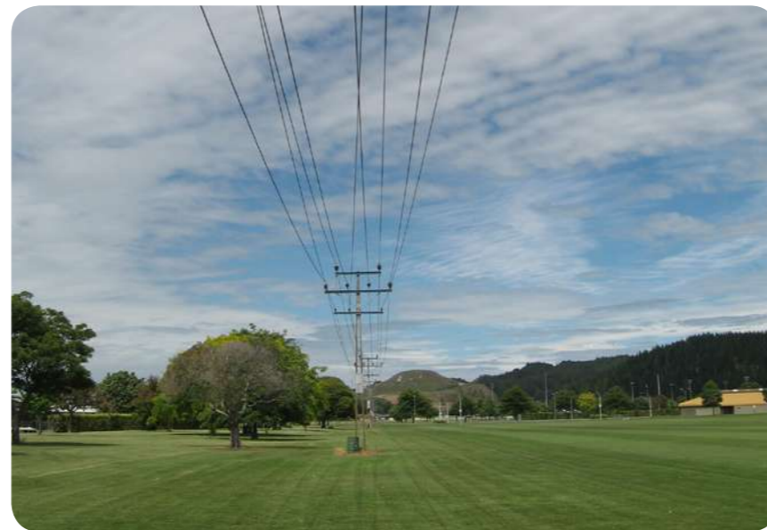
Overhead Lines through playing fields
